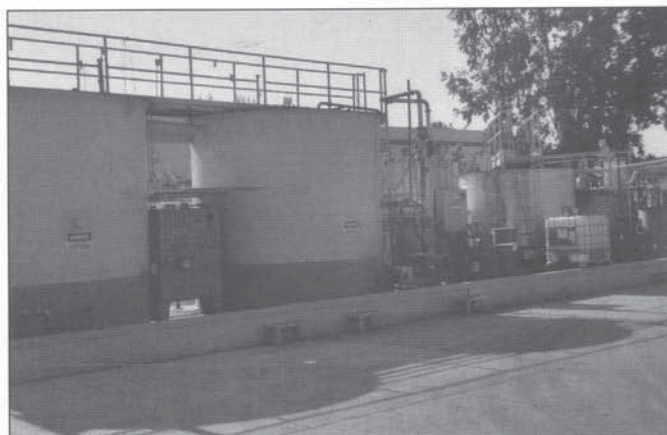
Waste water treatment system at Moorpark.
