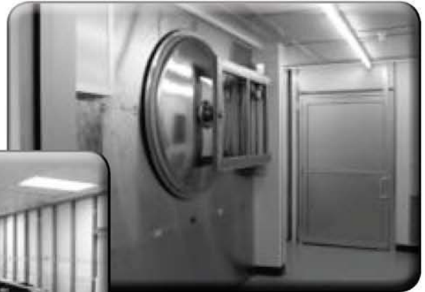
New 600 lbs Consolidated Dryer installed as part of expansion project.
