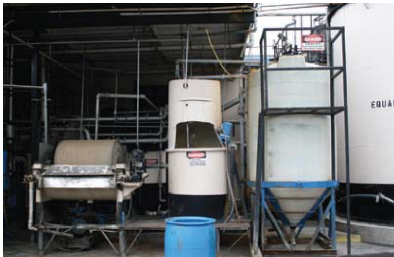
Chemical storage equipment near the wastewater-treatment area is marked with warnings to employees about confined-space restrictions.
