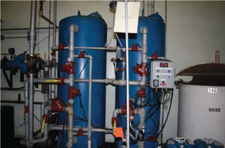
A view of water softening equipment
