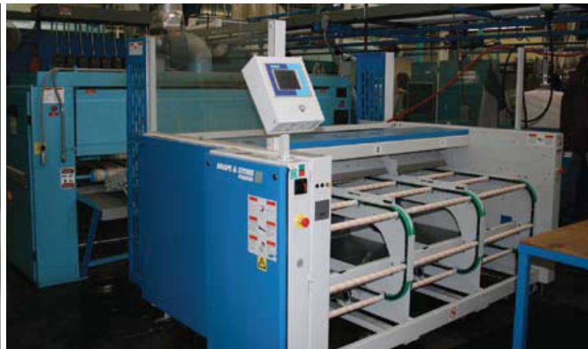
A Jensen stacking/storage machine sits at the end of the ironer.
