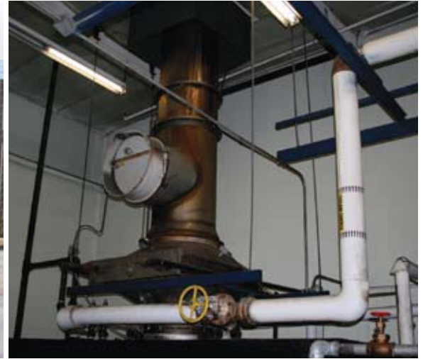
A stack economizer in the plant
