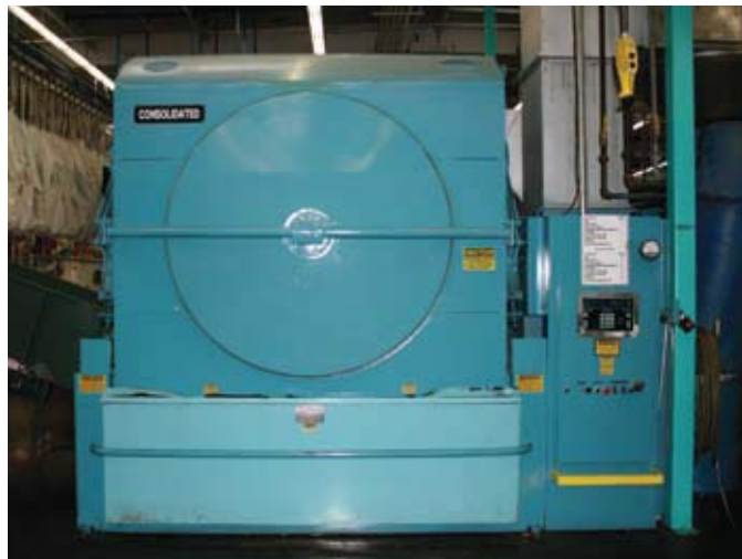
A CLM dryer in the wash aisle
